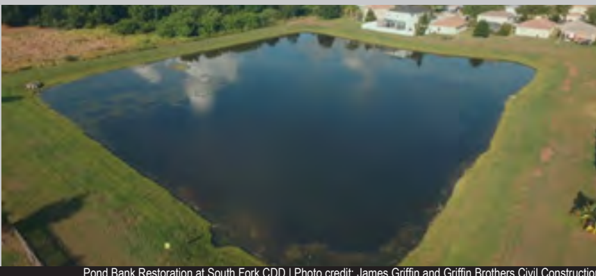
Pond Bank Restoration at South Fork CDD | Photo credit: James Griffin and Griffin Brothers Civil Construction
